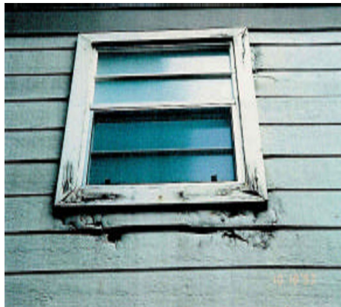
Poor flashing and sealing
