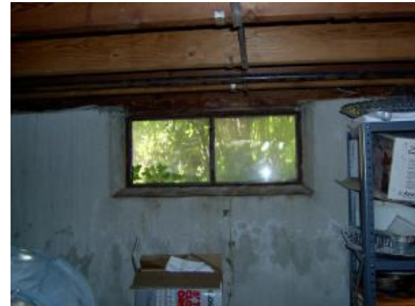
Single Pane Basement Window – Typically, an air sieve
